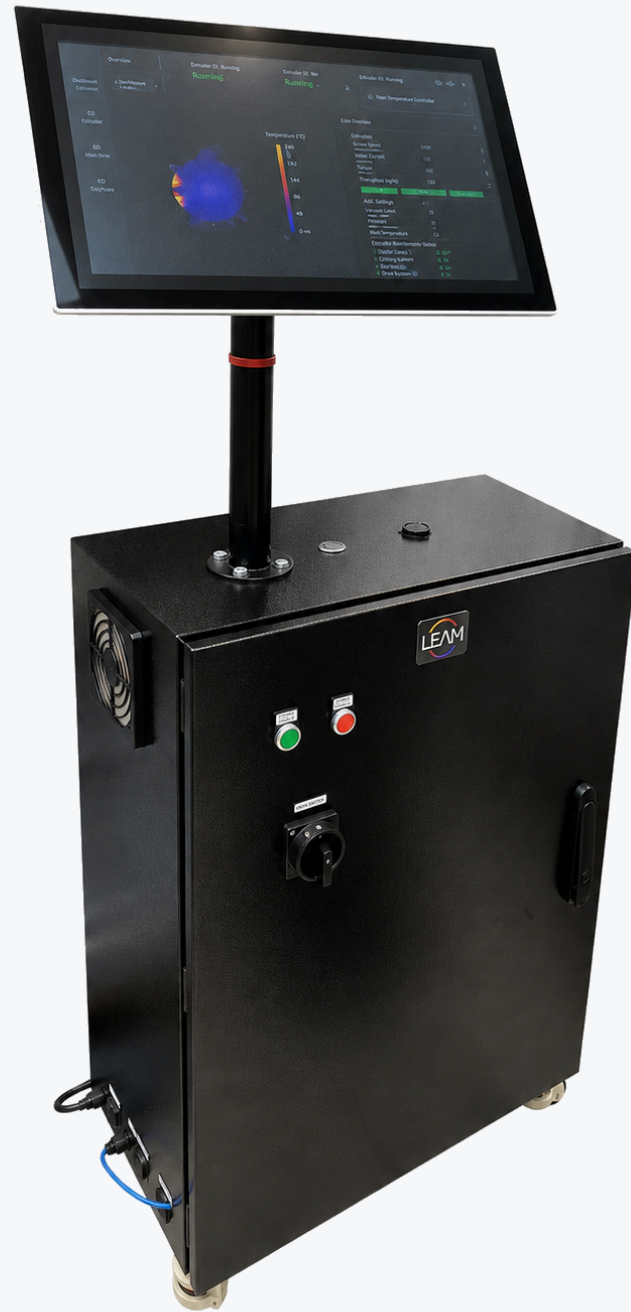
Electrical cabinet with HMI touchscreen and front controls.
